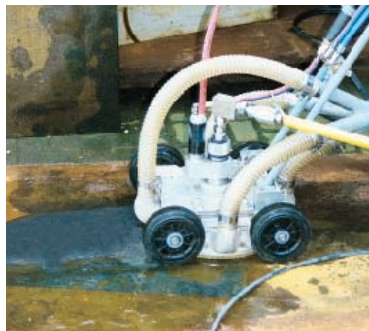
Derusting of bottom boards using a removal-suction tool and steel decoating with a rotating water jet tool
