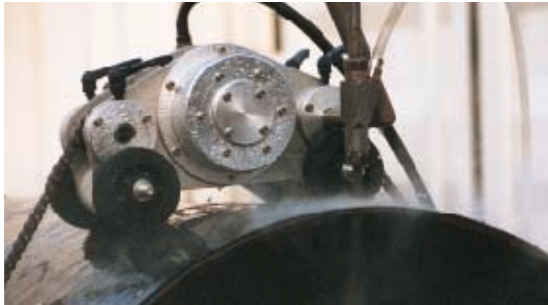
Demolition of rubber coated pipe elements using an abrasive water jet cutting unit
